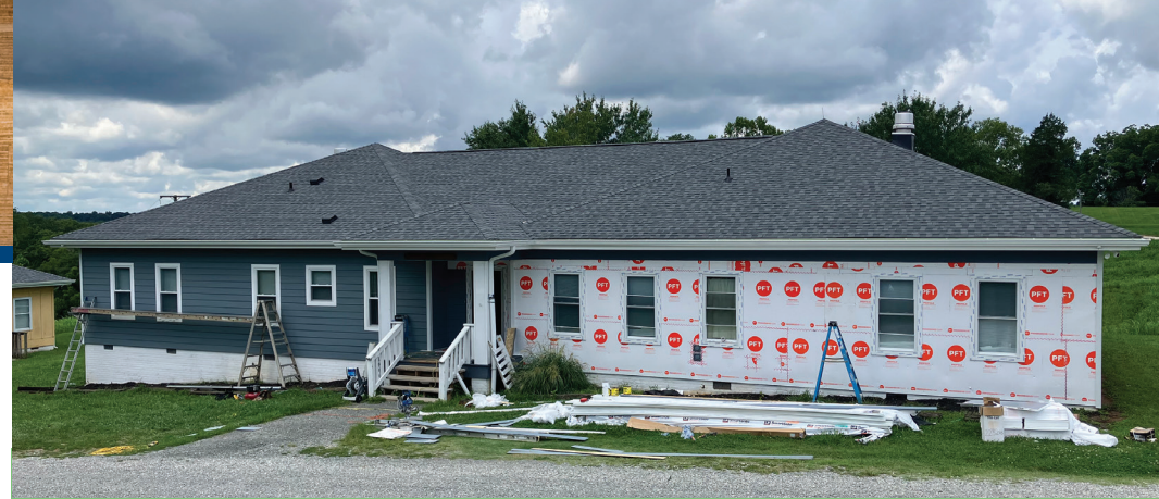
Siding, roofs, windows and decks were replaced on the residential cottages for youth living at Elk Hill.
